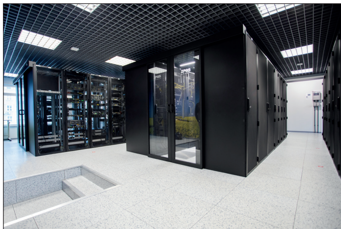
Data Center PSE - Bydgoszcz
